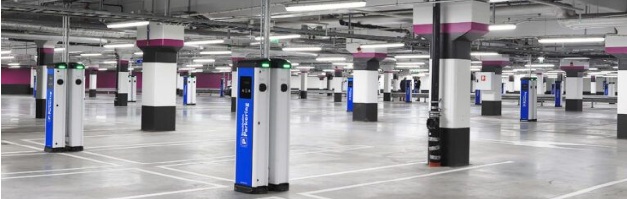
EV CHARGING IN BUILDING PARKING FLOOR
